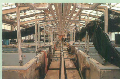
Primary stage rearing facilities for fry
